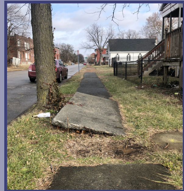
Dislodged sidewalk segment
