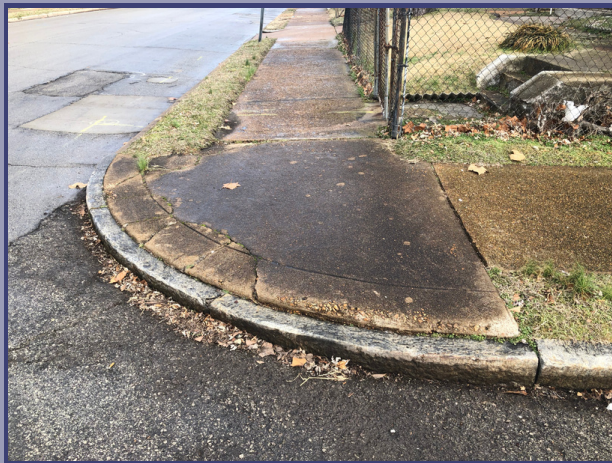
Curb at an intersection missing all ramps
