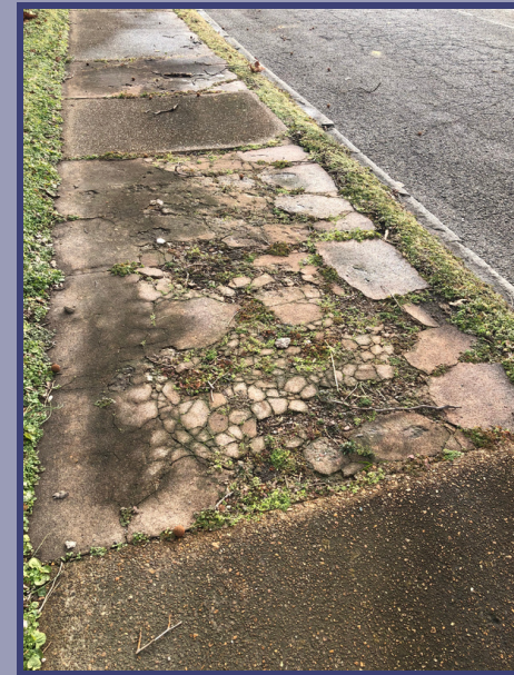
Weathered, crumbling sidewalk surface
