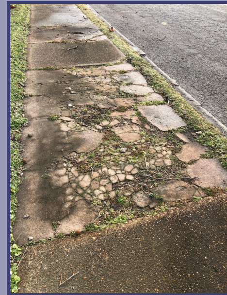
Weathered, crumbling sidewalk surface
