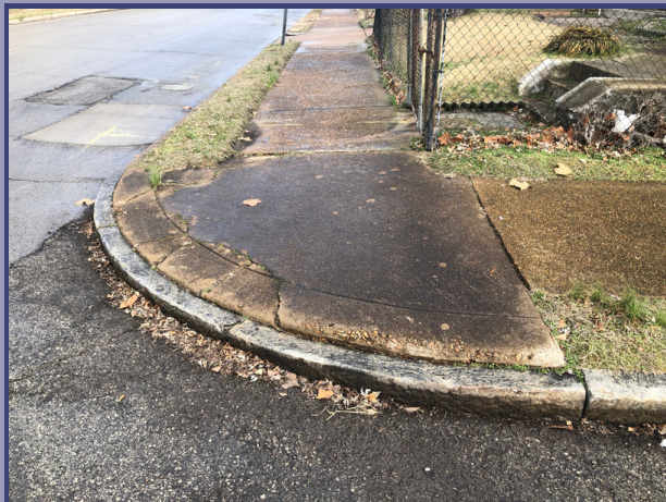
Curb at an intersection missing all ramps
