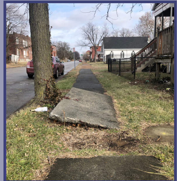
Dislodged sidewalk segment
